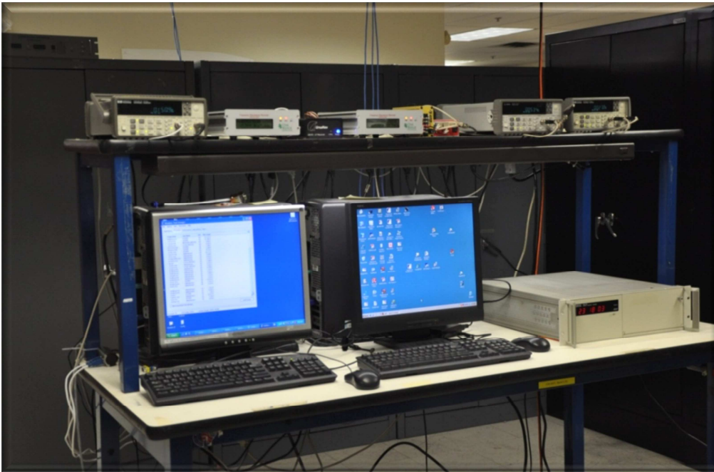
Figure 8: eLoran for SmartGrid trial set-up in Bedford, MA.
