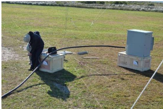
Figure 36. Heliac connected to the ATU
