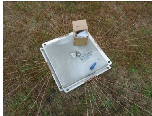
Figure 27. Ground radials attached to the base plate
