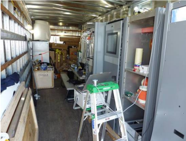
Figure 35. Positioning of the eLoran transmitter components
