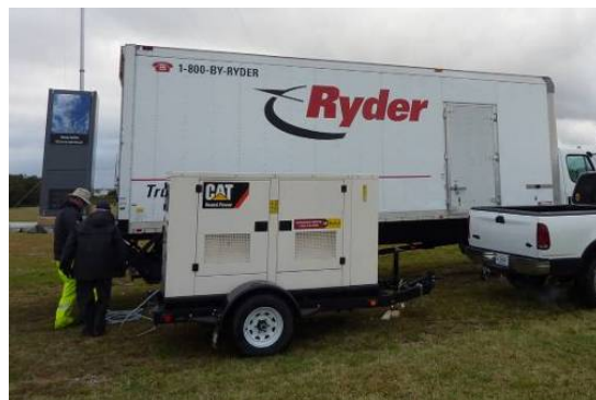
Figure 16. Caterpillar 220V, 20 kW diesel generator
