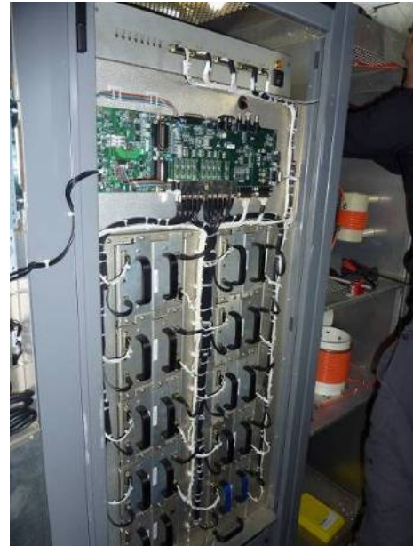
Figure 34. Setting-up the Nautel 50 kW transmitter
