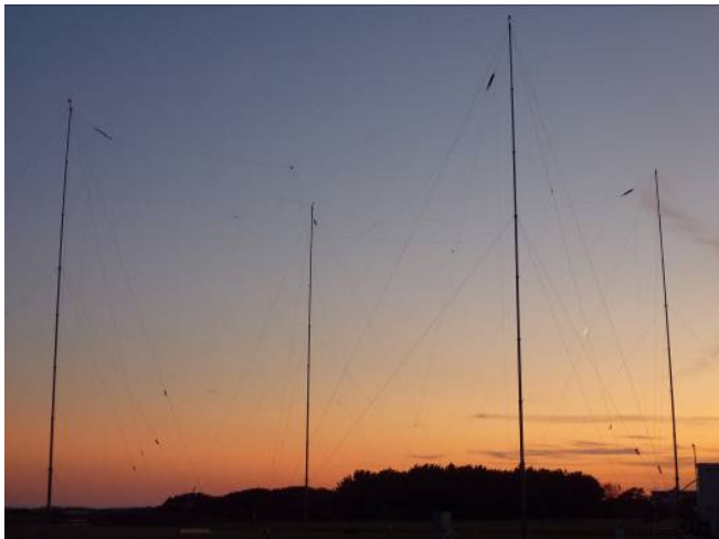
Figure 33. 21-m (70-ft) inverted cone antenna
